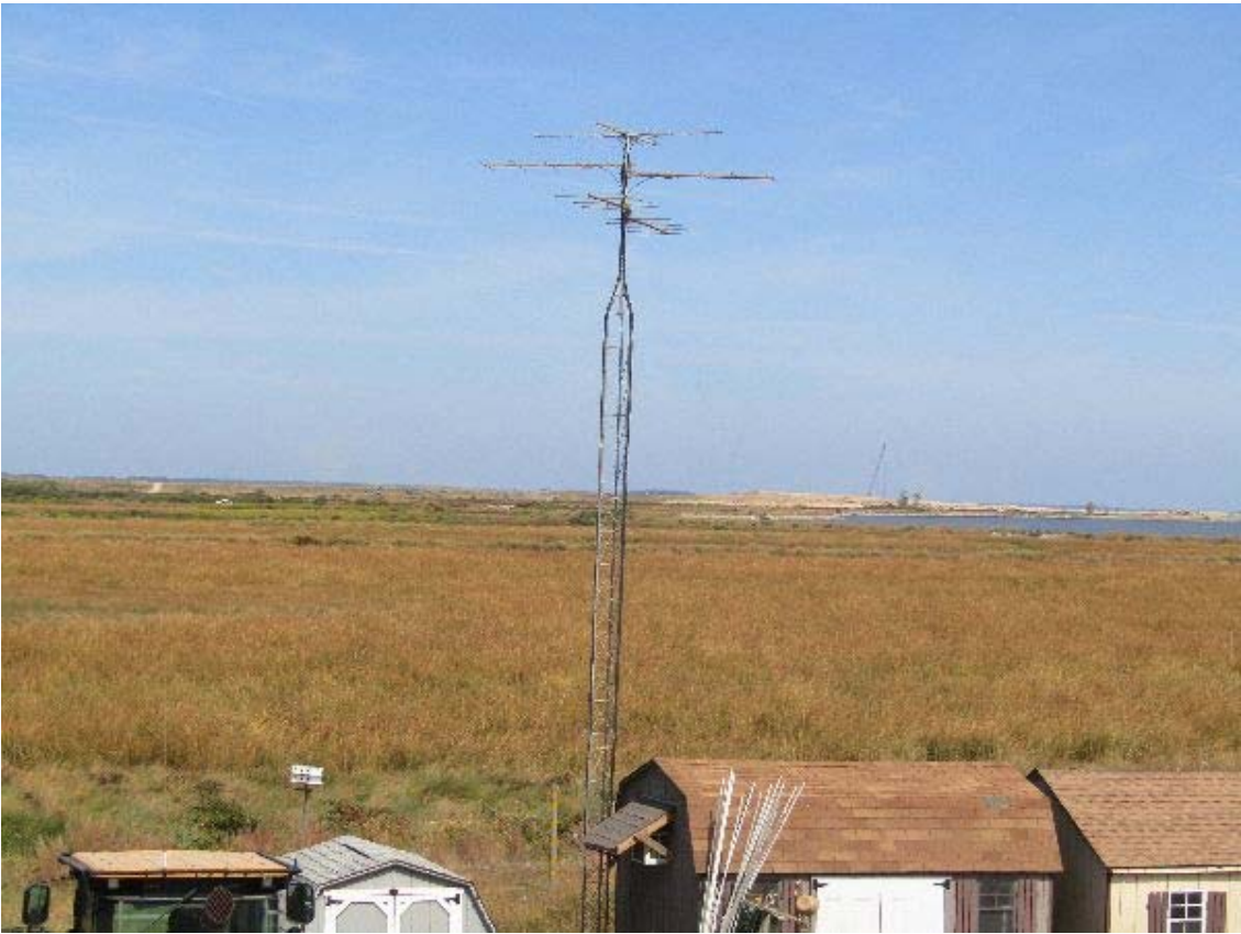
Motus Tower Installed on Poplar Island.
