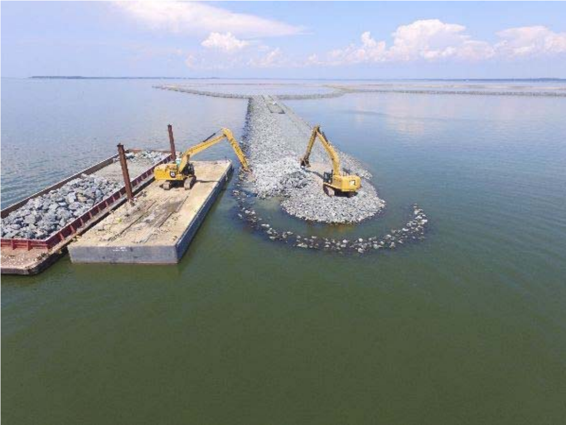
The Wesson Group LLC. placing armor stone behind the toe dike around the breakwaters of the open water embayment.
