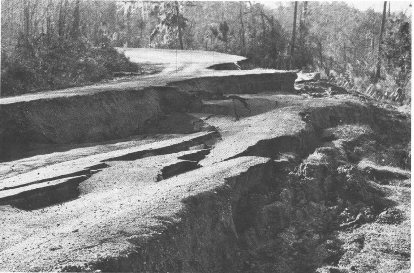
Figure 1.—Soil slippage is a severe limitation to local roads and streets in this area of Bayoudan clay, 5 to 40 percent slopes.
