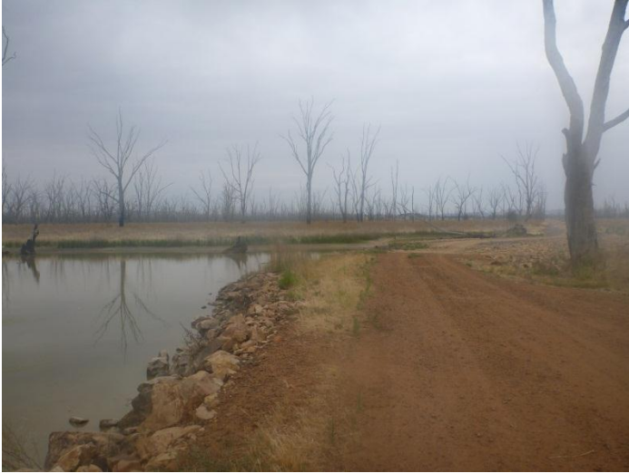
Fig. 3-20 The road embankment on Boggy Bridge Road, showing artificial water level on the Boggy Bridge Swamp side.
